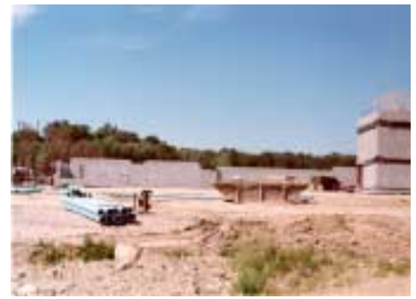
Walls on SB2 and HB stair tower This Photo from Horning Construction
