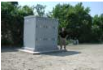
Switch Gear behind Youth Care Facility
