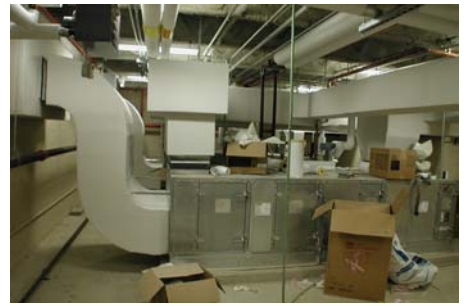
HG Mechanical Room
